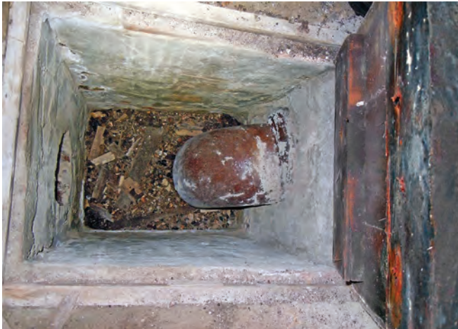
Ventilation chamber open
